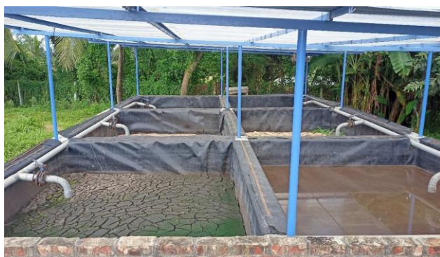
Figure 2: Sludge emptying and drying bed
