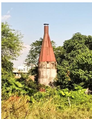
Figure 6 Incinerator in UAMCH premises
