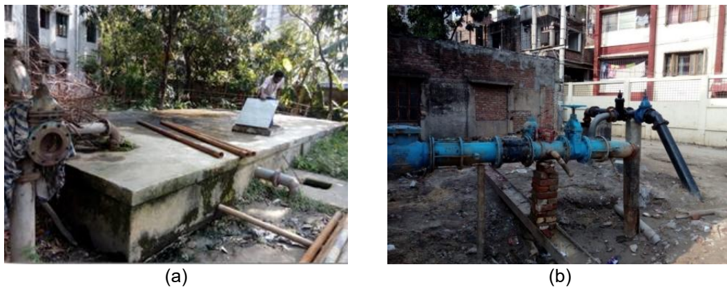
Figure 2 (a) Water reservoir. (b) WASA water pump.
